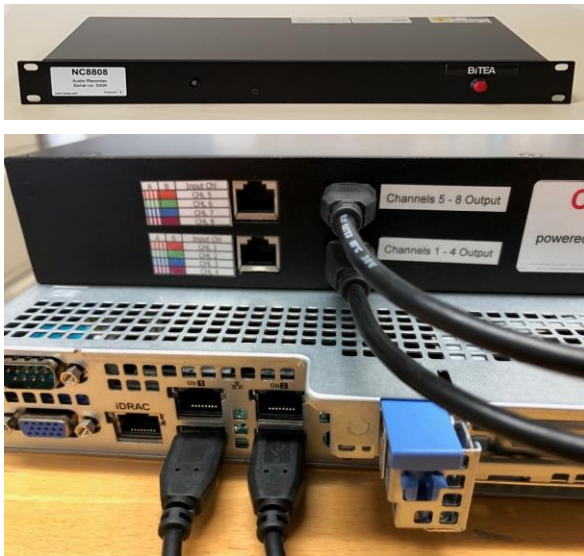
Designed from an original concept for the Radio Communications Department of Dorset Police
